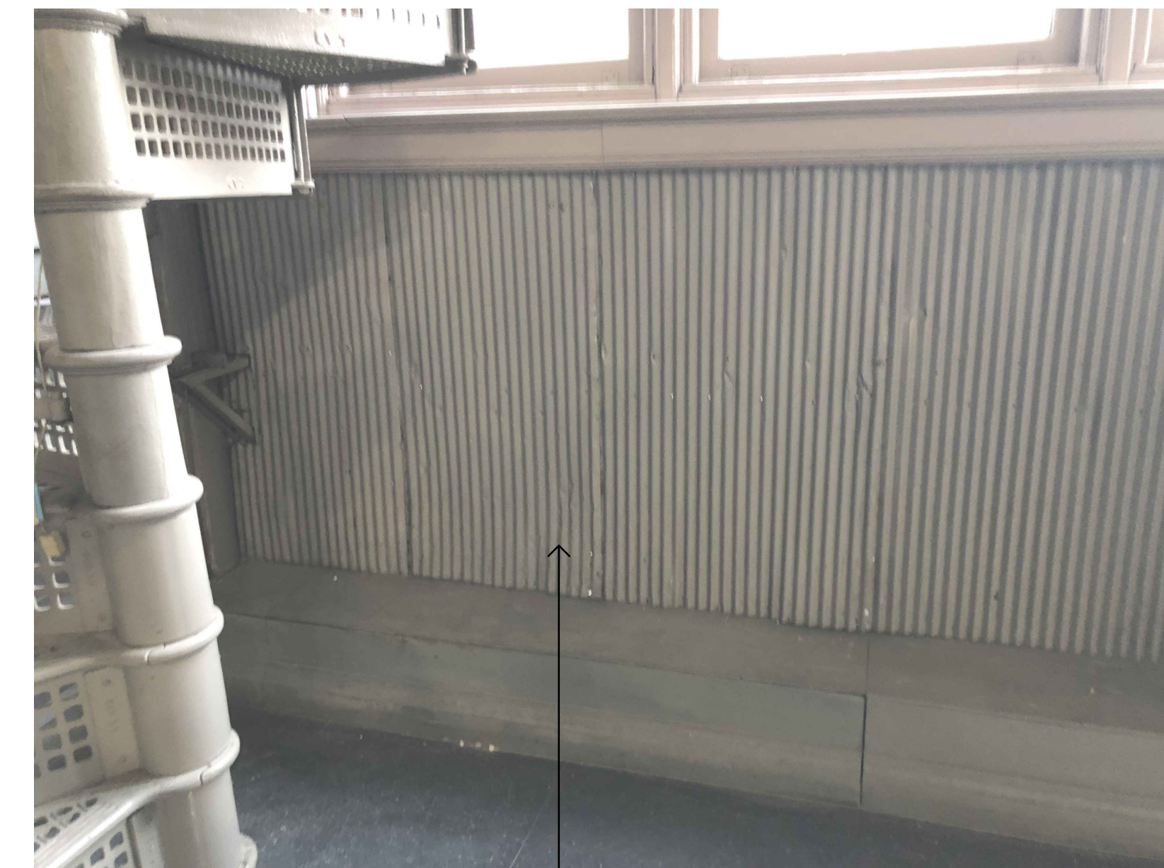
REMOVE AND REPLACE CORRUGATED METAL PANEL IN THIS ENTIRE BAY TRUSS 3 TO 5 ON THE WEST ELEVATION PROFILE TO MATCH EXISTING; PAINT NEW PANELS
