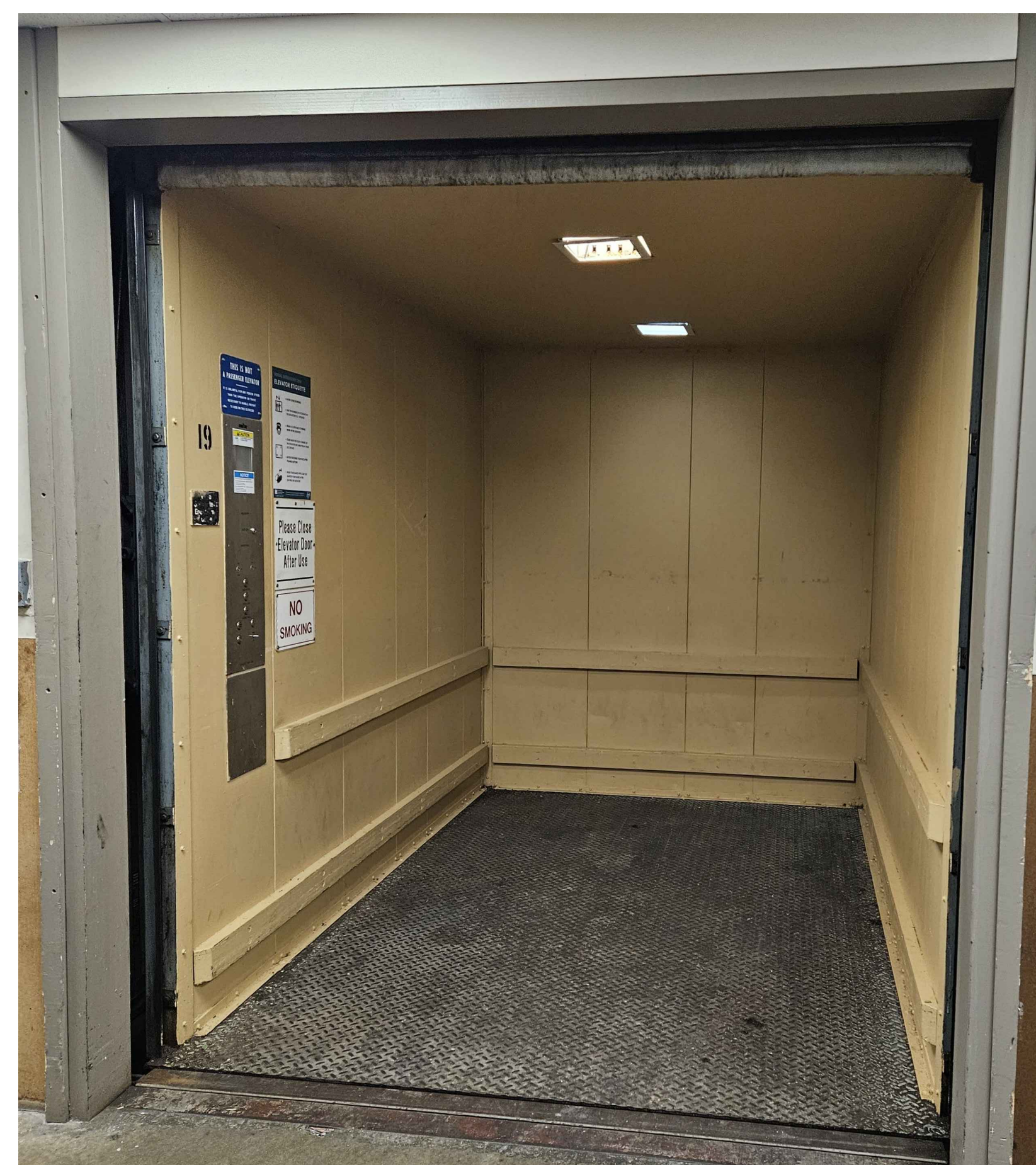
6 ELEVATOR #19 CAR LIGHTS PHOTO SCALE: NTS
