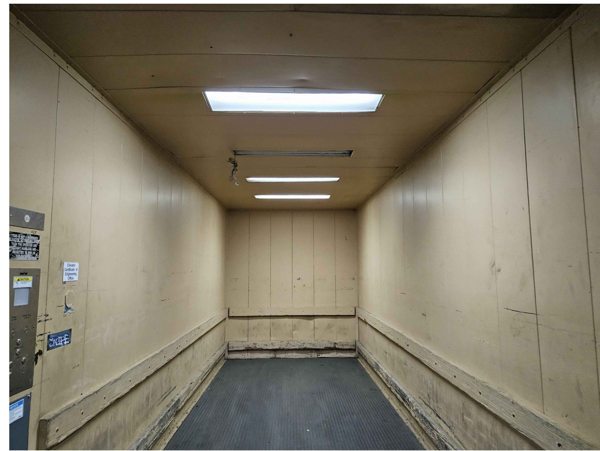
3 ELEVATOR #28 CAR LIGHTS PHOTO SCALE: NTS
